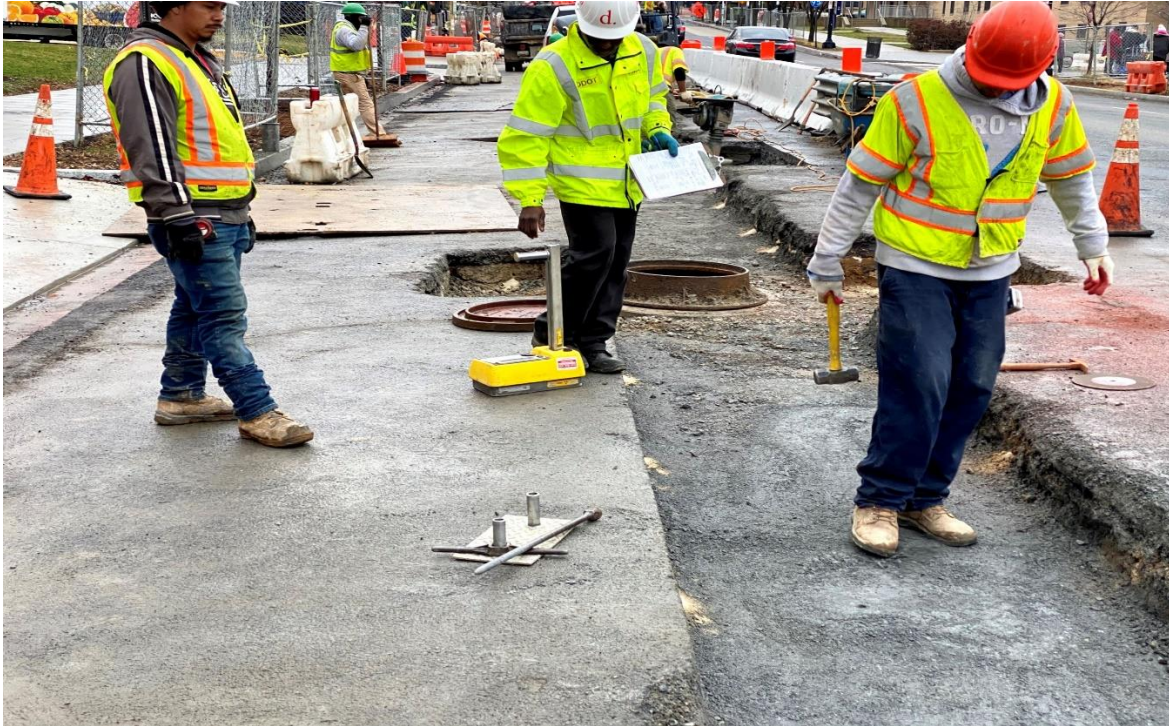
01/04/2020- Moisture-Density Test Activity at West side curb lane, NJ Ave. NW near Sta. 114+25.
