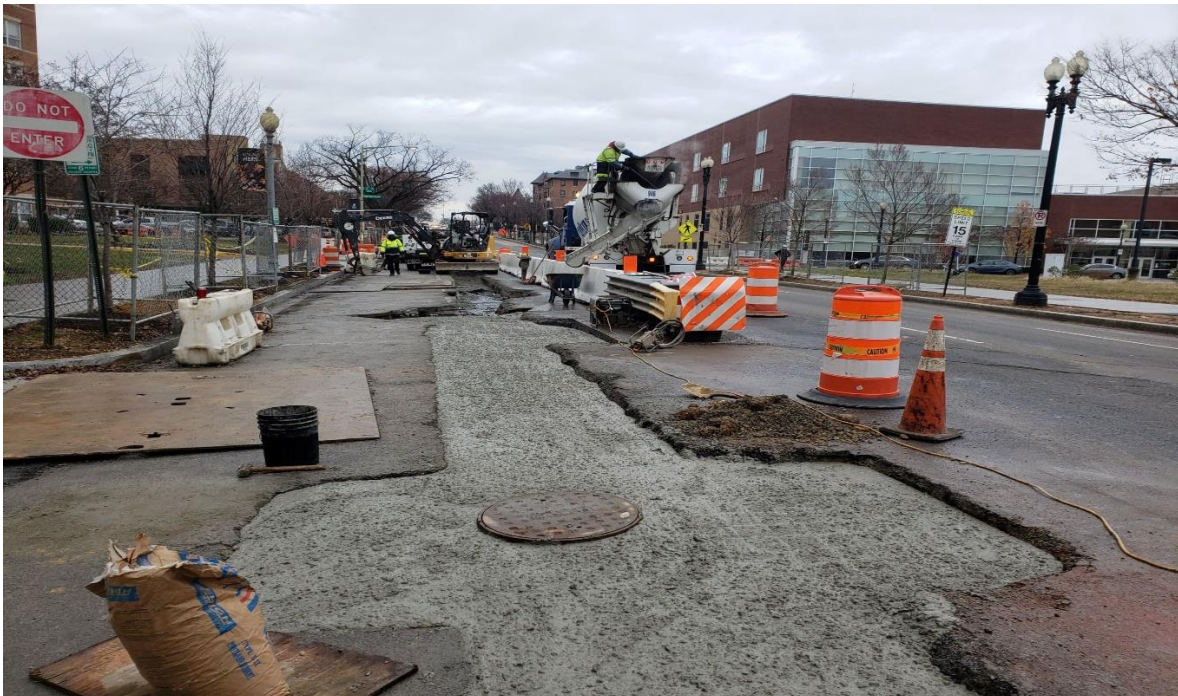
01/04/2020- Repairs to PCC base over utility trenches at NJ Ave. NW between K & L St. NW. (North View)
