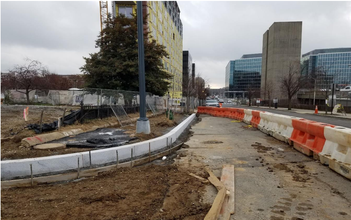
12/31/2019- Granite straight and circular Curb installed at East side 2 nd and I St. NW (South view)
