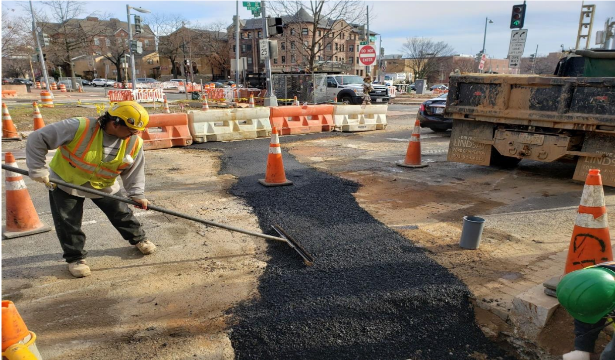
01/02/2020 – Temporary Asphalt Placement at across 3 rd St NW over sewer pipe trench Picture No. 8
