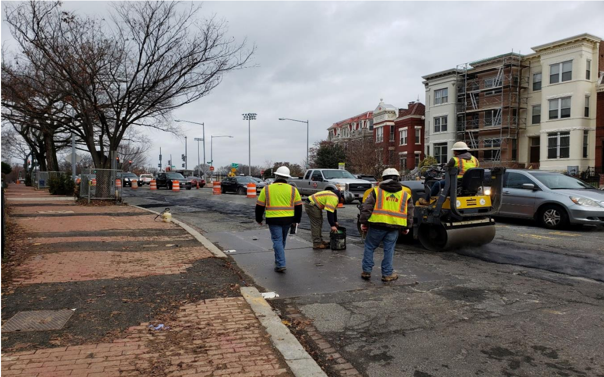
12/31/2019- Compaction to temporary asphalt placed on PCC base along the trench line between Morgan & N St. NW.
