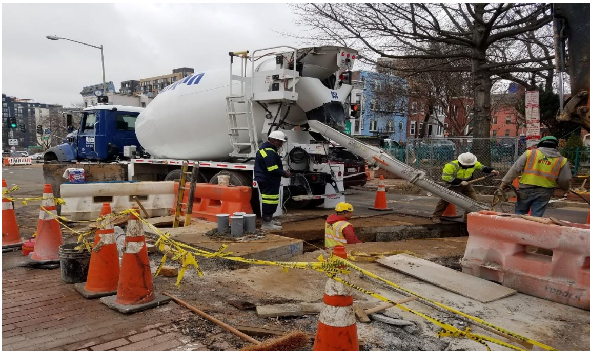
12/31/2019 – Concrete pouring to encase the pipe between MH-C2 to CB-D near 3 rd & M St. NW.
