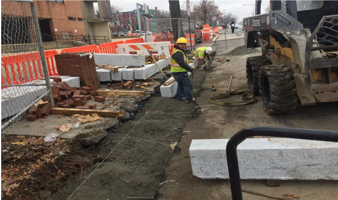
12/31/2019- Setting of granite straight curb along West side of NJ Ave. NW b/n Pierce and NY Ave Picture No. 2
