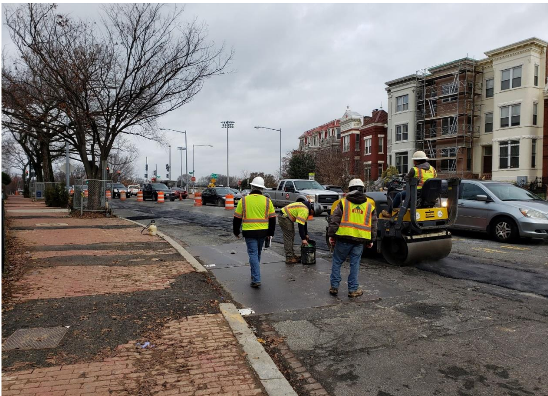
12/31/2019- Compaction to temporary asphalt placed on PCC base along utility trench line between N St & Morgan St. NW.
