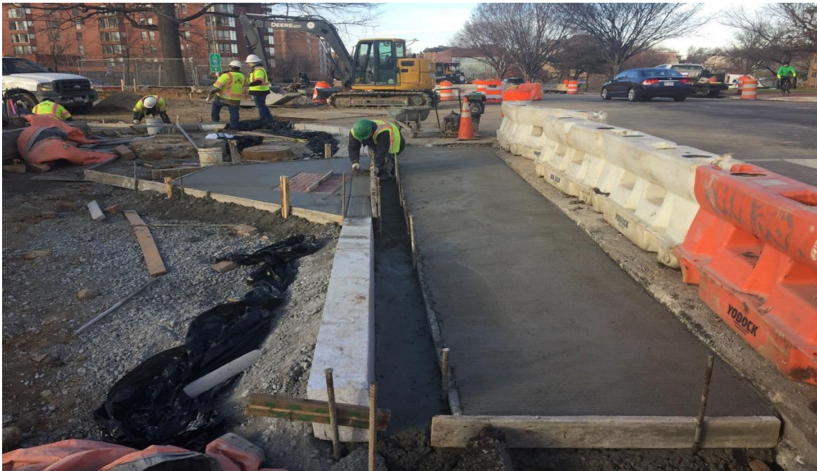
01/02/2020- Wheelchair ramp construction at SW corner of New Jersey Ave. & I St. NW.
