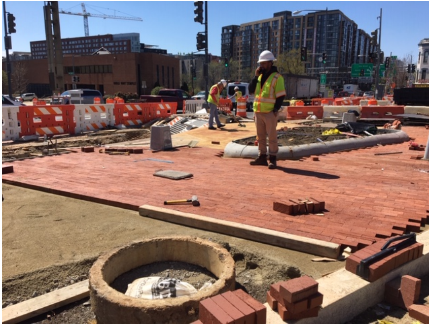
Picture No. 1: 03/30/2020 - Installation of brick sidewalk at the NE corner of NJ Ave and NY Ave intersection – island (West View)
