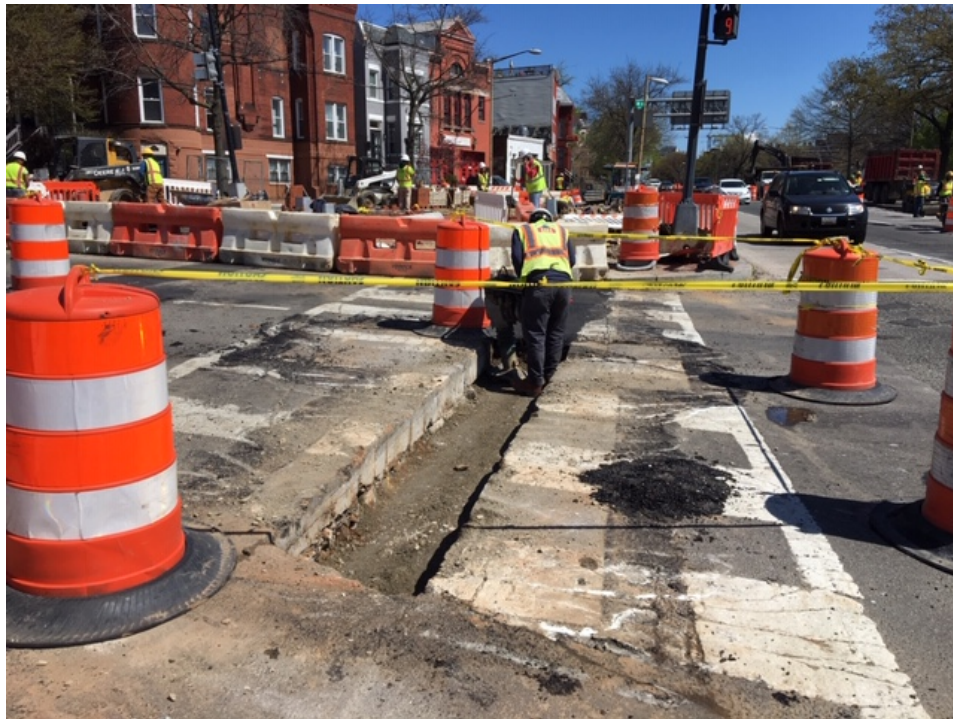
Picture No. 3 - 03/30/2020 – Compaction of GAB material over utility trench at the NE corner of NJ Ave and NY Ave intersection – island (West View)
