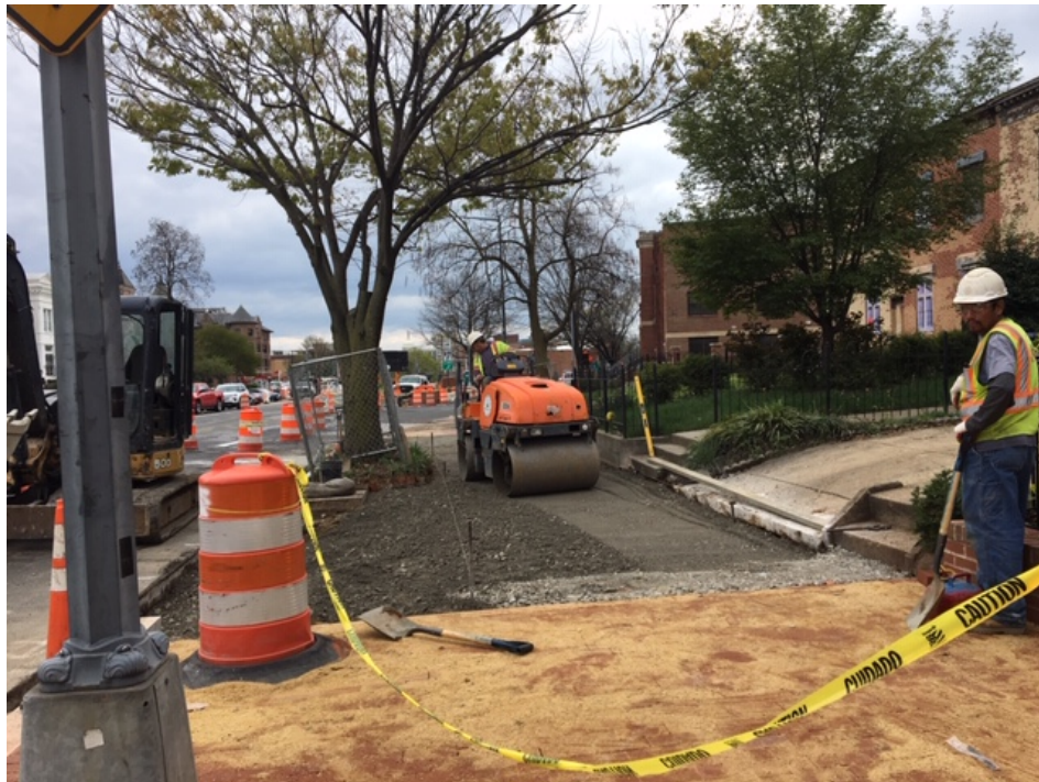
Picture No. 9 - 04/01/2020 – Compaction of GAB material on the sidewalk and driveway at NJ Ave and N St. (South View)
