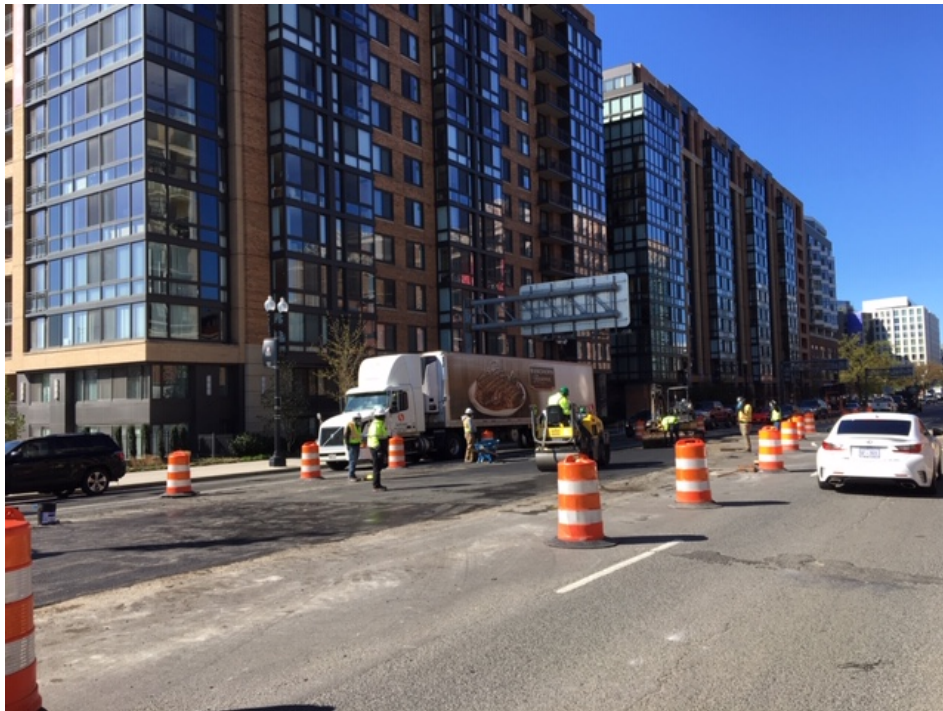
Picture No. 13 - 04/03/2020 – Installation of temporary asphalt on the median along NY Ave. between 4 th St and 5 th St. (West View)
