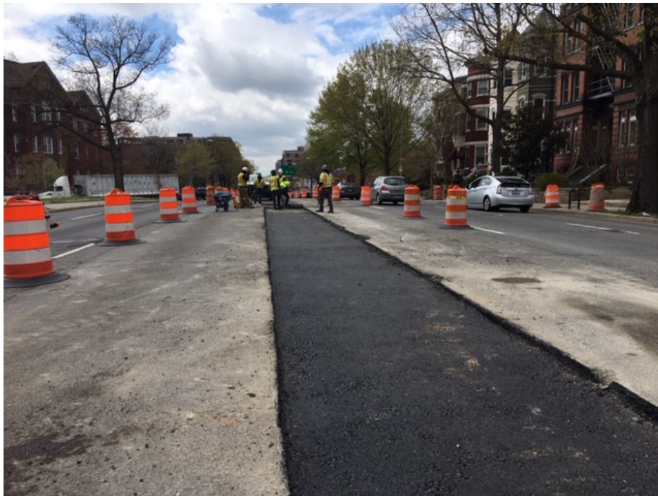
Picture No. 8 – 04/01/2020 – Installation of temporary asphalt in the median along NY Ave between 1 st St. and NJ Ave. (East View)
