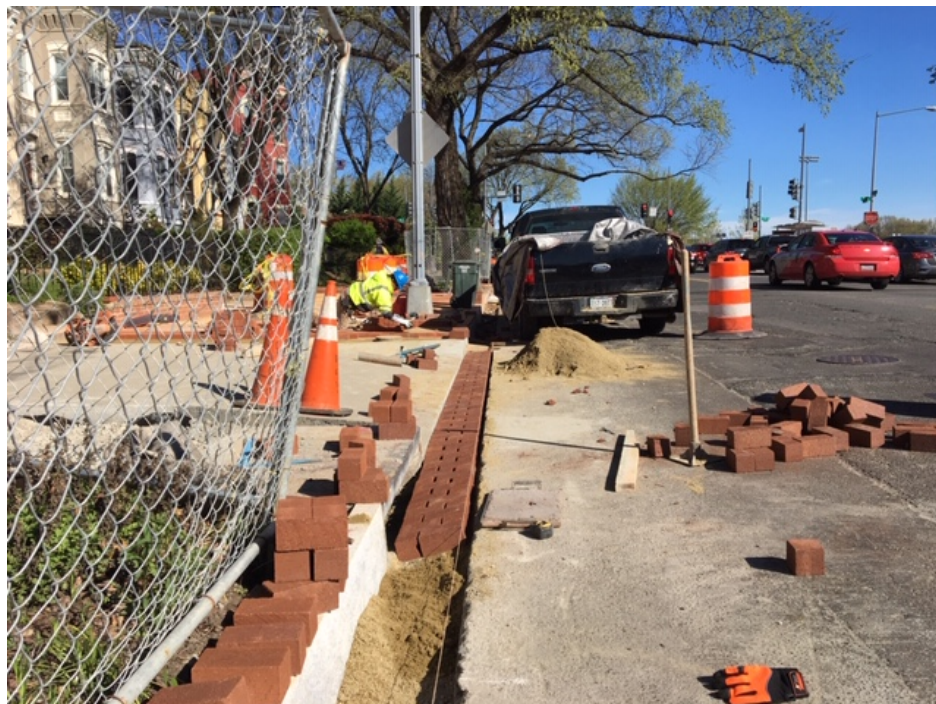
Picture No. 12 – 04/03/2020 – Installation of brick gutter along NJ Ave SB at the intersection of NJ Ave and N St. (North View)
