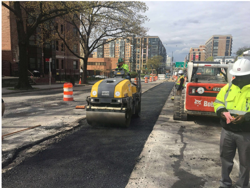
Picture No. 5 - 03/31/2020 – Installation of temporary asphalt along NY Ave between 1 st St and NJ Ave (West View)
