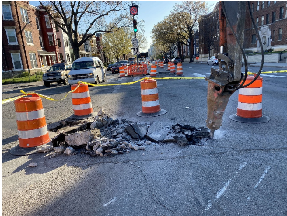
Picture No. 11 - 04/02/2020 – Excavation for traffic signal conduit work at the intersection of 1 st St and NY Ave. (East View)
