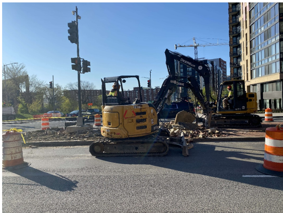
Picture No. 10 – 04/02/2020 – Removal of median along NY Ave between 4 th St and 5 th St (South View)
