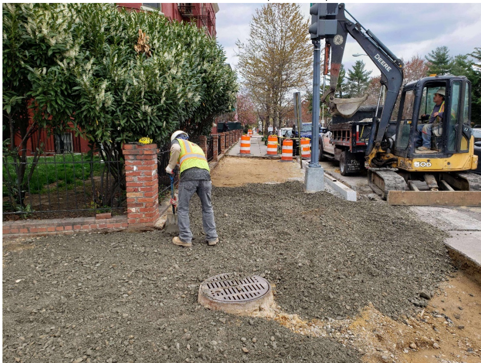
Picture No. 4 - 03/31/2020 – Placement of GAB material on the sidewalk at the intersection of N St. and NJ Ave (West View)
