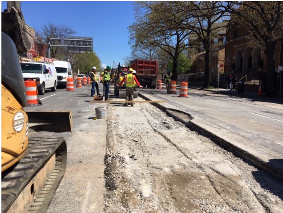
03/30/2020 – Compaction of GAB material in the median along NY Ave between 1 st St. and NJ Ave. (West View)
