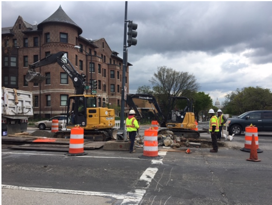
Picture No. 7 - 04/01/2020 – Removal of median at the intersection of NY Ave and NJ Ave (South View)
