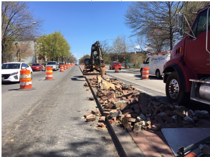
Picture No. 2 - 03/30/2020 – Removal of median along NY Ave between 1 st St. and NJ Ave. (West View)
