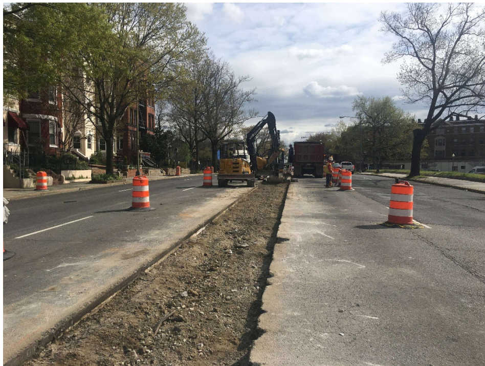
Picture No. 6 - 03/31/2020 – Median preparation along NY Ave between 1 st St and NJ Ave (East View)
