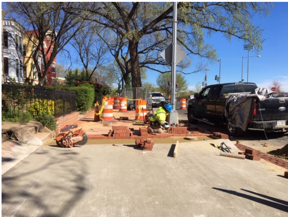
Picture No. 14 – 04/03/2020 – Installation of brick sidewalk across Morgan St on SB NJ Ave. (North View)
