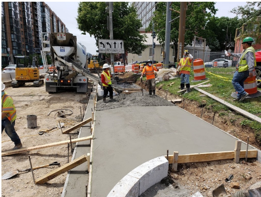
Picture No. 4 – 05/19/2020 – Concrete pour underway at NY Ave. between 3rd St. and 4th St. NB (East View)
