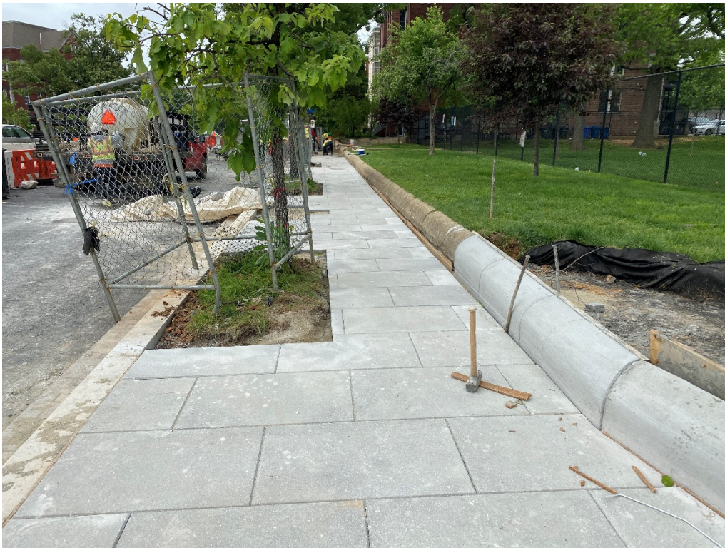
05/20/2020 – Block paver sidewalk installation along north side of NY Ave between First St and Kirby St. (West View)
