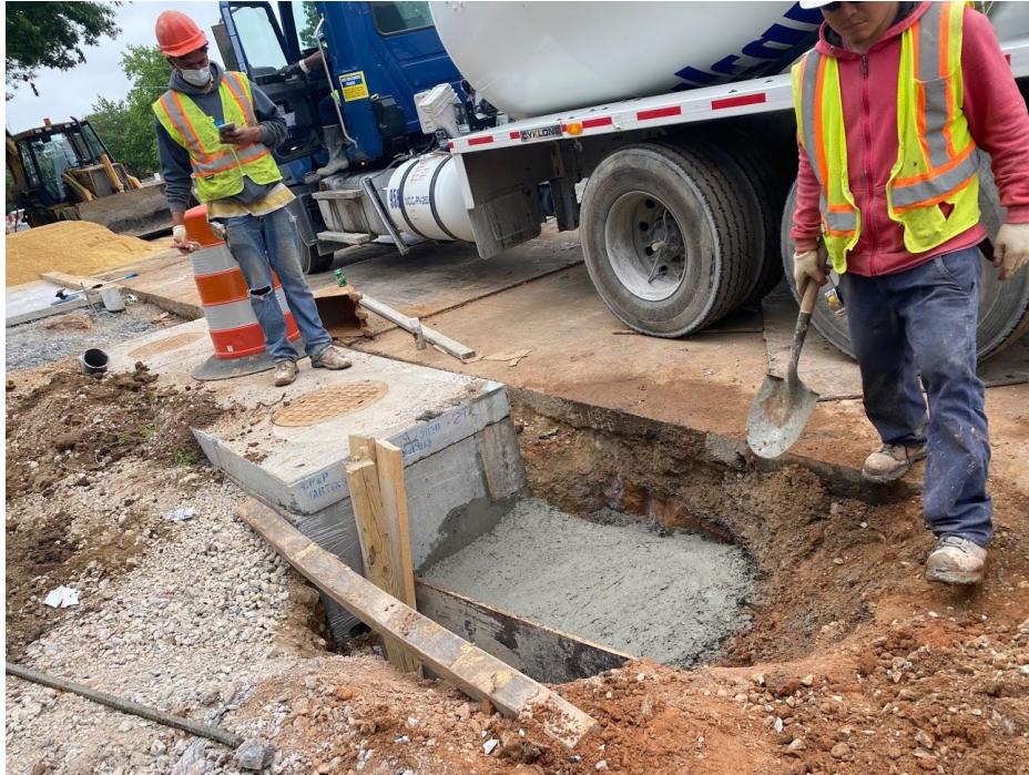
Picture No. 3 - 05/18/2020 – Connect pipe encased with concrete at NY and Kirby St. NW for CB-AA.
