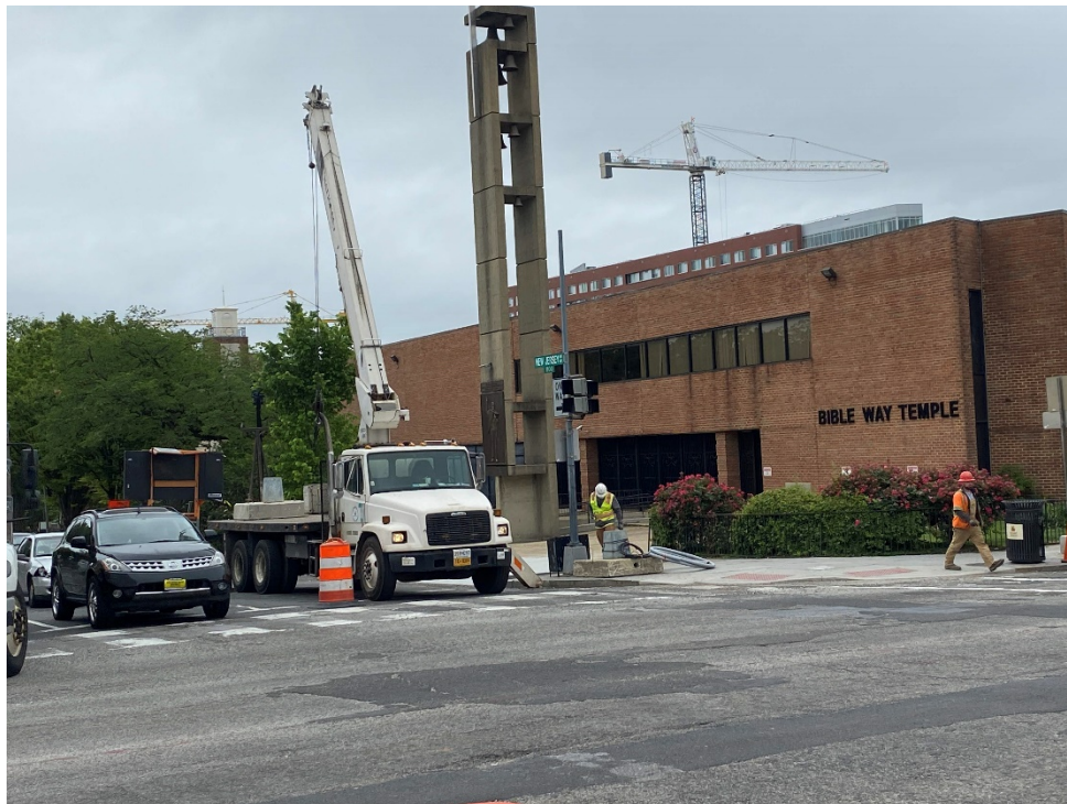
Picture No. 10 – 05/21/2020 – Traffic light pole transfer from one foundation to another at SW corner of NJ and NY Ave. (South View)
