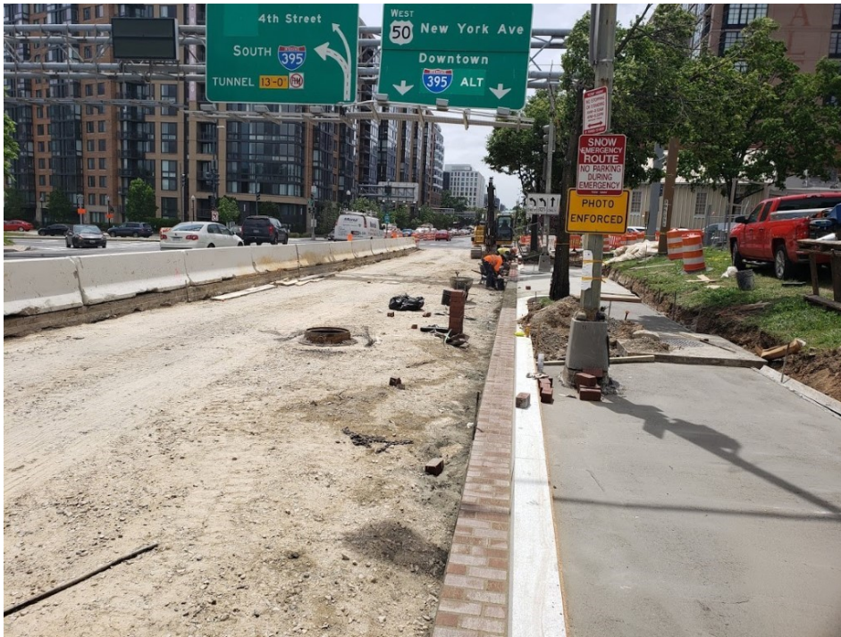
Picture No. 7 – 05/20/2020 – Placed brick gutter at NY Ave. between 3rd St. and 4th St. NB. (West View)
