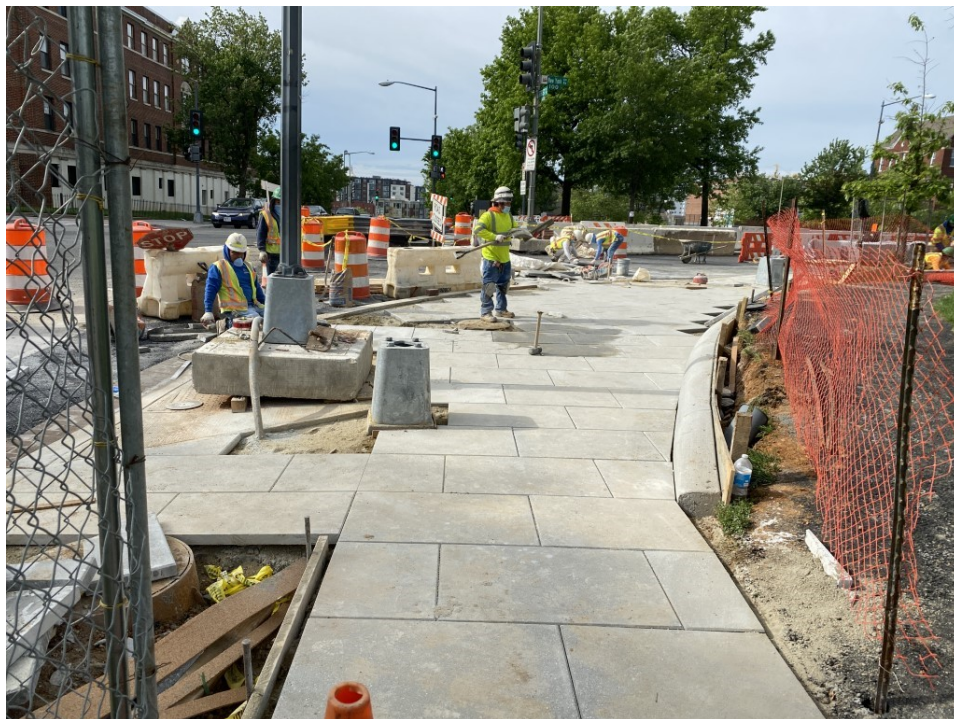
Picture No. 6 – 05/19/2020 – Block Paver sidewalk installation at NW corner of NY Ave and 1st. St. NW (South view)
