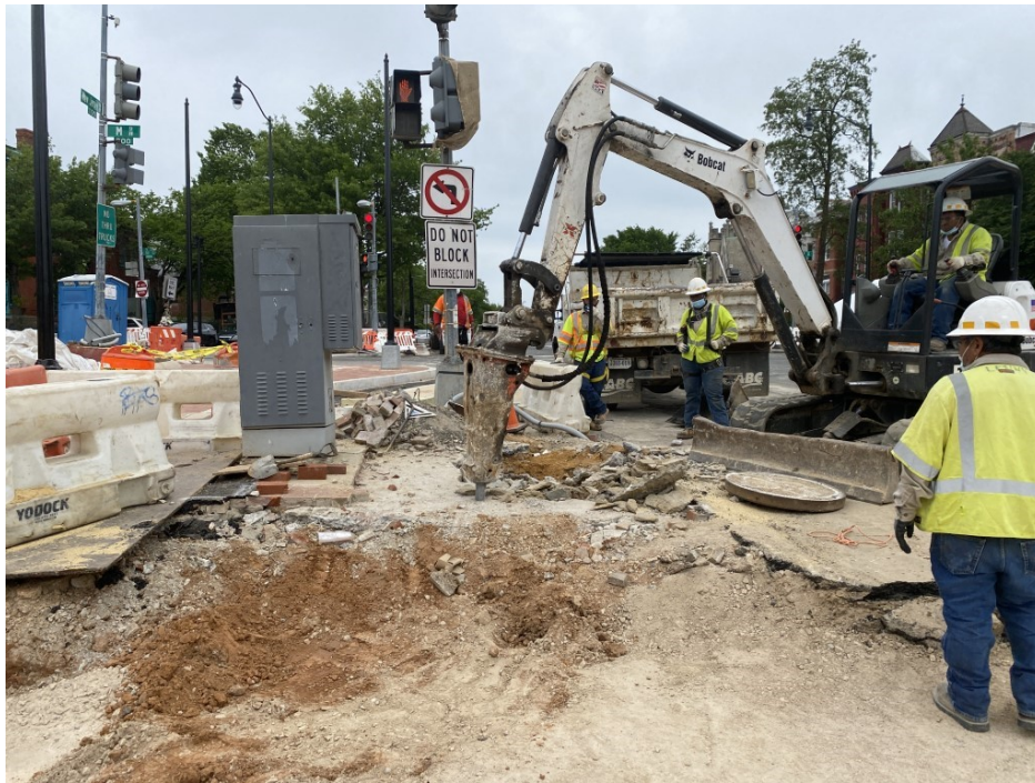
Picture No. 5 – 05/19/2020 – Pepco contractor demolition of electrical manhole at NJ Ave. at NY Ave and NJ Ave intersection (East View)
