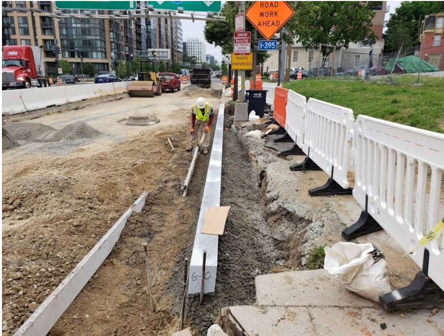
Picture No. 1: 05/18/2020 – Furnished and installed granite curb at NY Ave. between 3rd St. and 4th St. NB. (West View)
