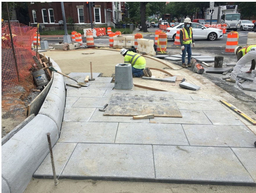
Picture No. 2: 05/18/2020 – Placing concrete block sidewalk near NW corner of NY Ave. and First St (East View)
