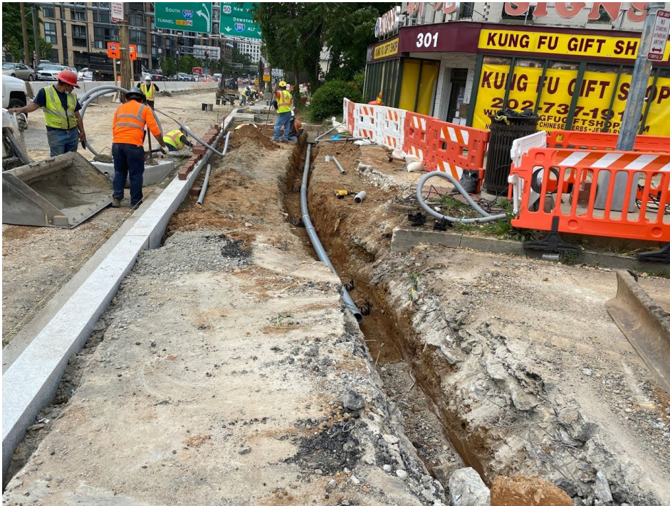
Picture No. 8 – 05/20/2020 – PVC conduit pipe installation near NW corner of NY Ave and 3 rd St. NW. (West view)
