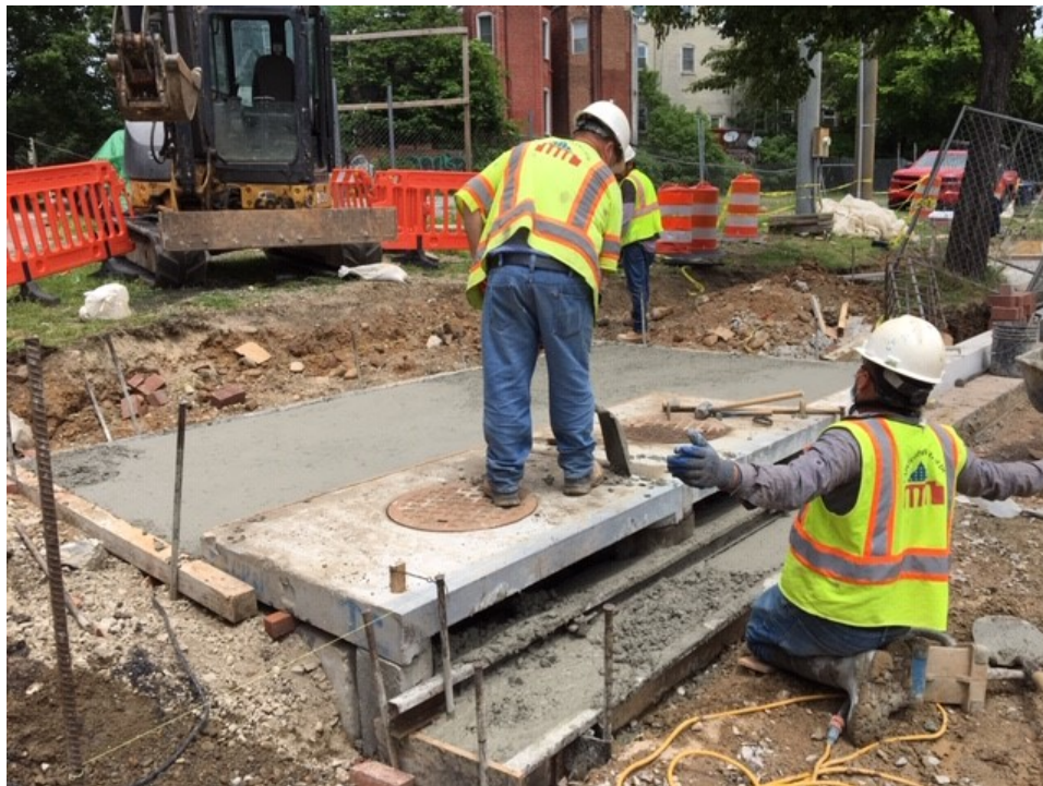
Picture No. 12 – 05/21/2020 – PCC installed at the double catch basin location at Sta. 320+24 along the sidewalk (Northeast View)
