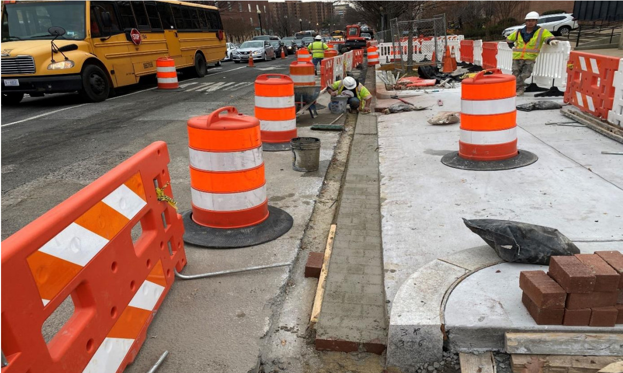
01/24/2020- Brick gutter construction along West side of NJ Ave. NW b/n Pierce & NY Ave. (South view) Picture No. 10
