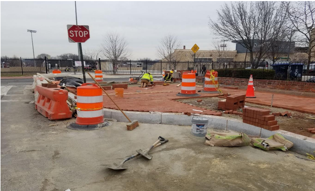
01/22/2020- Brick sidewalk construction at East side of 3 rd St. near N St. NW. (NE view)
