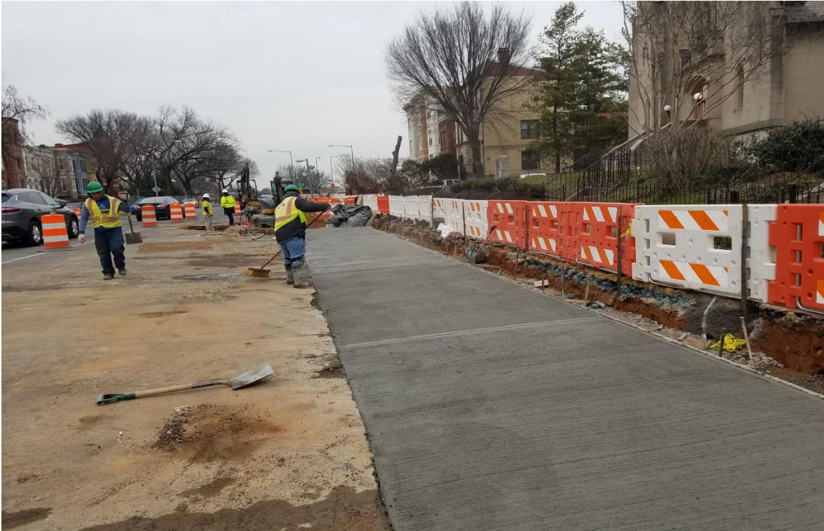
01/23/2019- PCC Base constructed at East side of NJ Ave. b/n Morgan St and M St. NW. (North view) Picture No. 6
