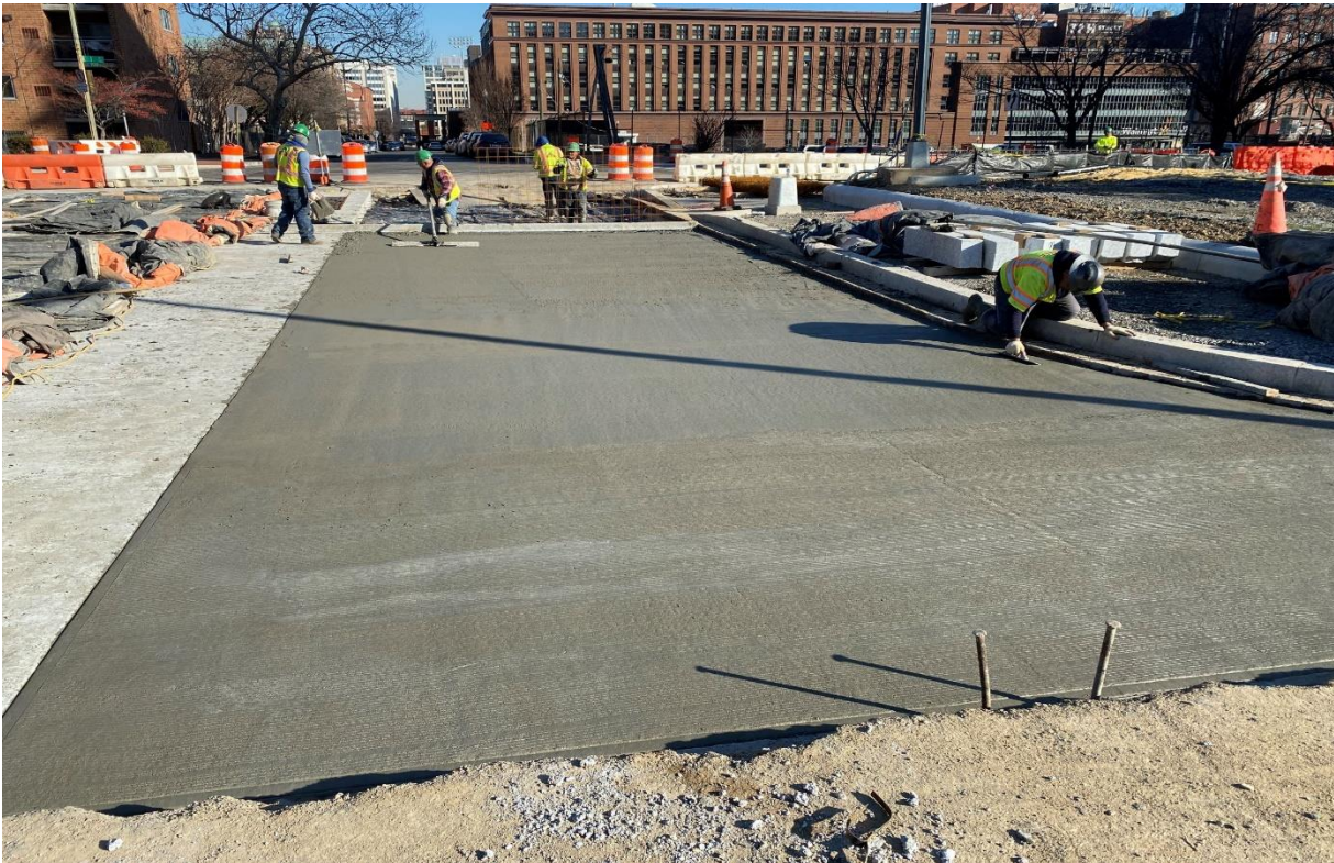
01/21/2020 - PCC Base construction at South side of I St. NW between NJ Ave. & 2 nd St. NW. (East view)
