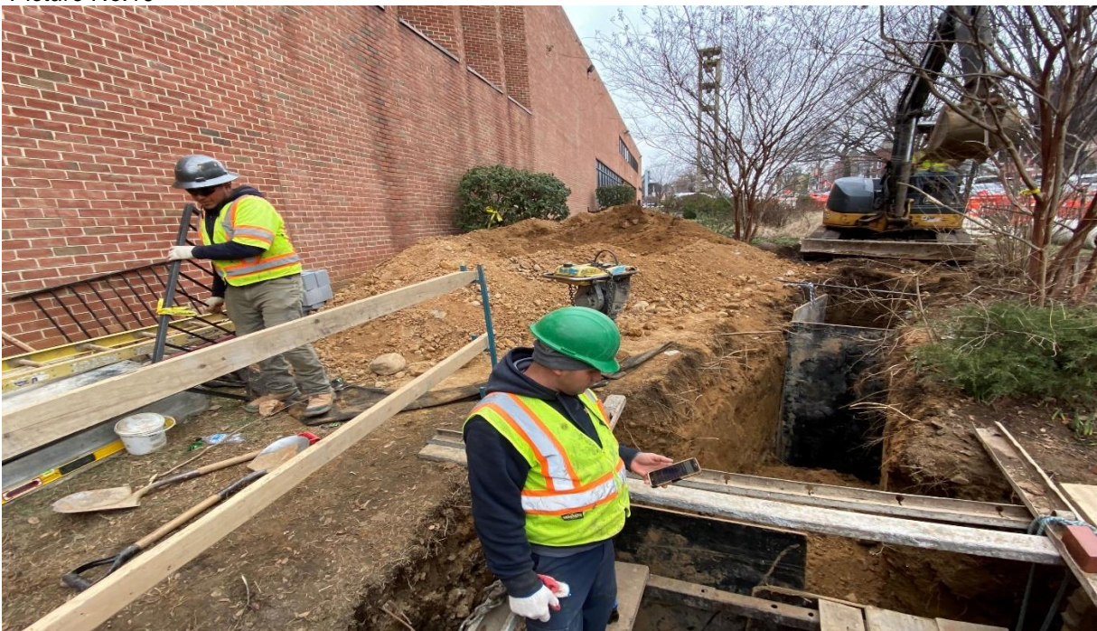
01/24/2020- Excavation for sewer pipe at West side of NJ Ave. b/n Pierce & NY Ave. (North View)
