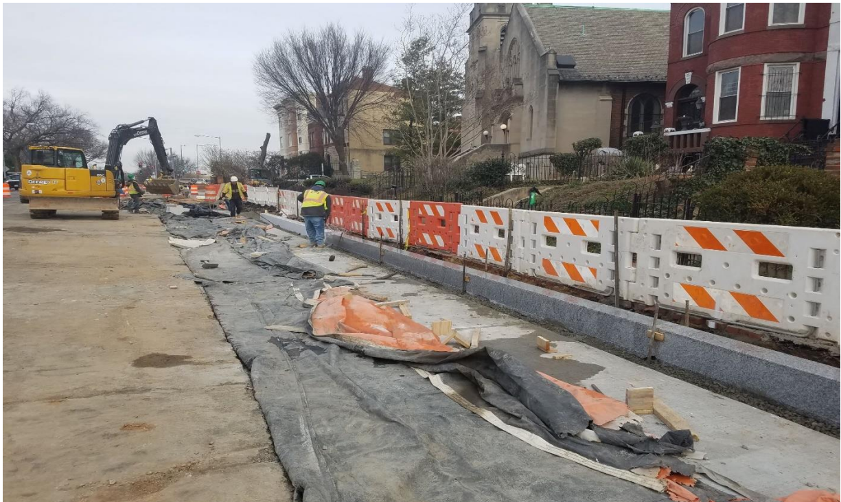
01/24/2020- Granite curb set at East side of NJ Ave. NW between M & Morgan St. NW. (NE view)
