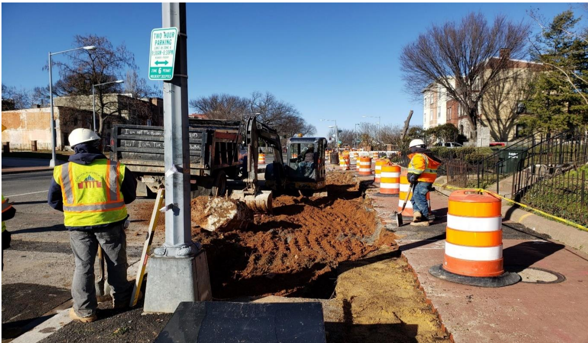
01/21/2020- Sidewalk excavation at East side of NJ Ave. NW between Morgan & N St. (N. view)
