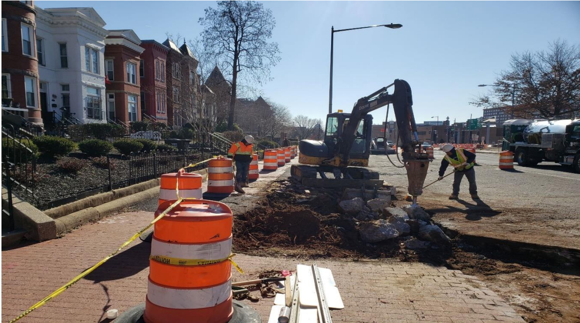
01/21/2020- Excavation for sidewalk and curb at East side of NJ Ave. between Morgan & M St. (S. view)
