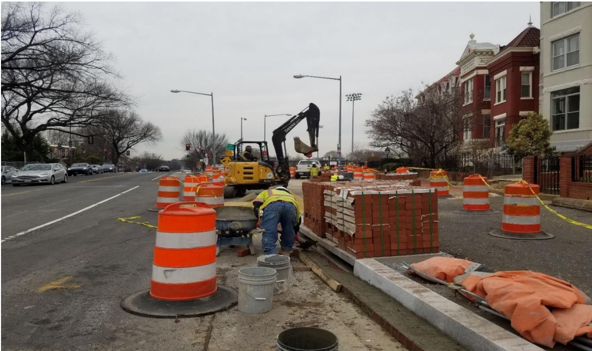
01/23/2020- Brick gutter construction at East side of NJ Ave. NW between M & Morgan St. NW.
