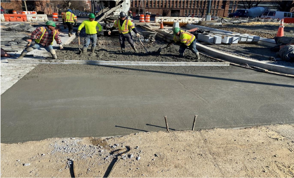
01/21/2020 – PCC Base construction at south side of I St. NW between NJ Ave. & 2 nd St. (East View) Picture No. 3
