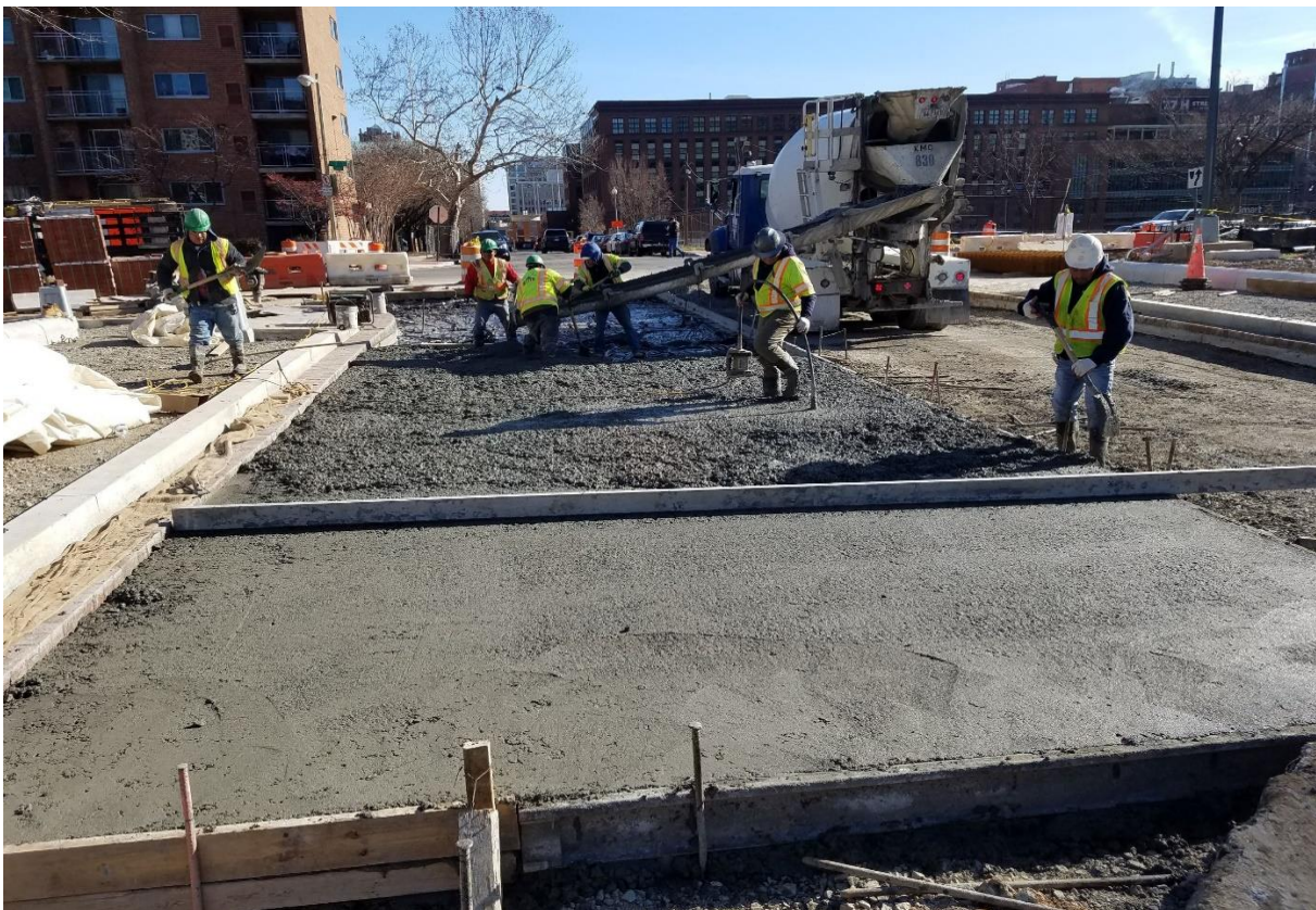
01/17/2020- PCC Base construction at I St. NW between NJ Ave. & 2 nd St. NW. (East view)
