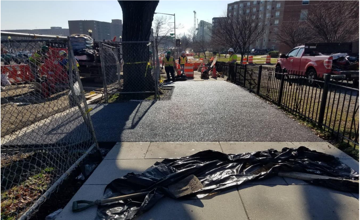
01/15/2019- Flexi pave for sidewalk at west side of NJ Ave. b/n L & Pierce St. NW. (South view) Picture No. 6
