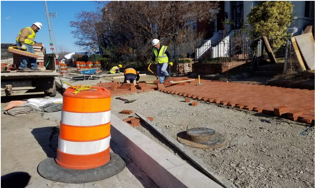
01/16/2020- Brick sidewalk construction at East side of 3 rd St between Morgan & N St. NW. (NE View)
