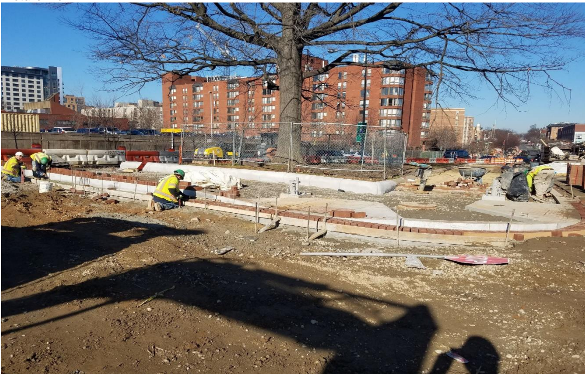
01/15/2020- Brick gutter construction at N side of I St. between NJ & 2 nd St. (North view)
