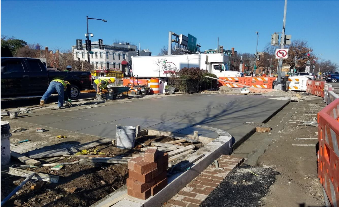
01/15/2020- Repairs to Driveway at West side of NJ Ave. NW at N. side of Bible church. (N. view) Picture No. 4
