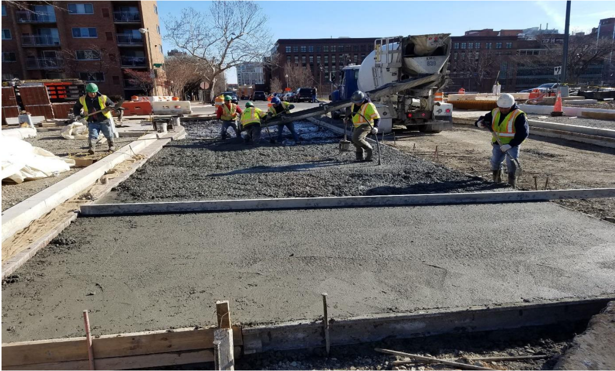
01/17/2020- PCC Base Construction at I St. between NJ Ave. & 2 nd St. NW. (East view)
