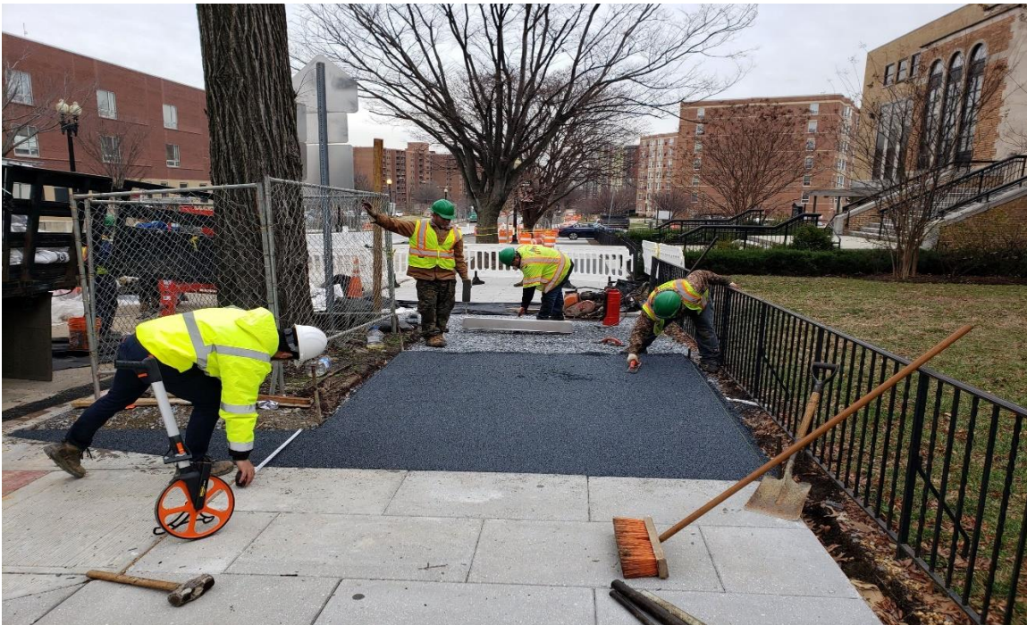
01/13/2020 – Flexi paving for the sidewalk at West side of NJ Ave. NW. b/n Pierce St. L St. NW (S. view)
