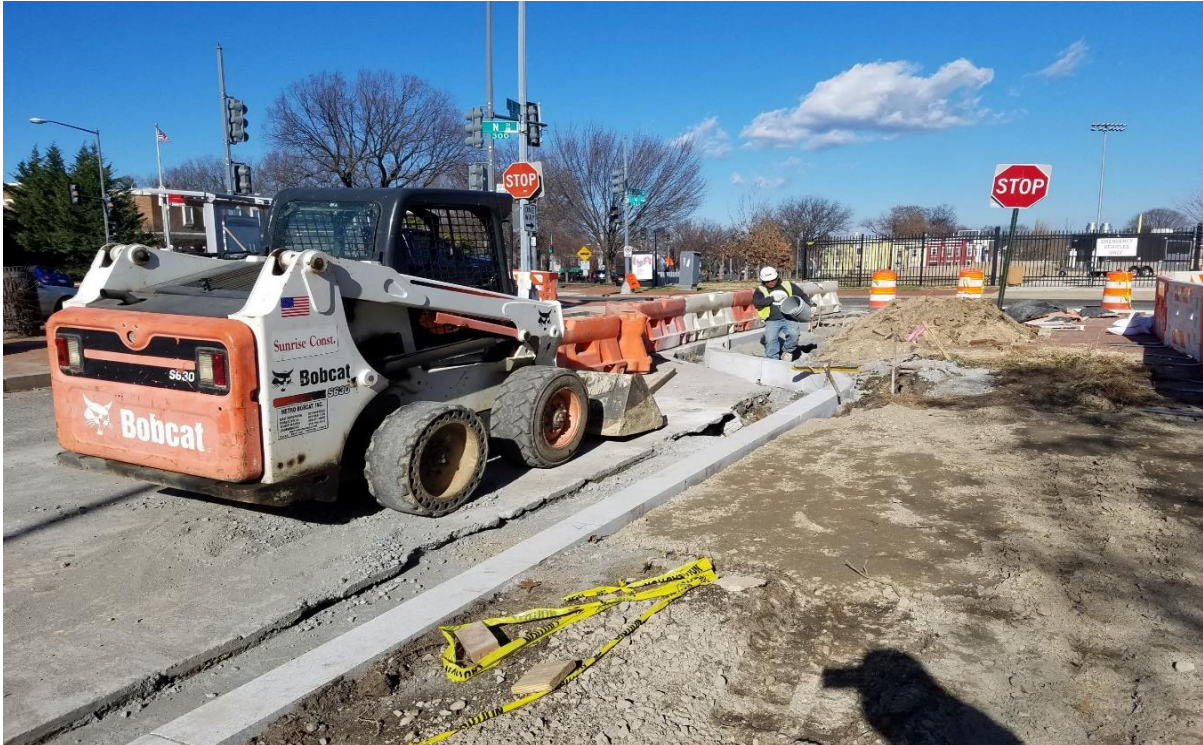
01/16/2020 – Furnished and set granite curb at East side of 3 rd St. near N St. NW. (North view)
