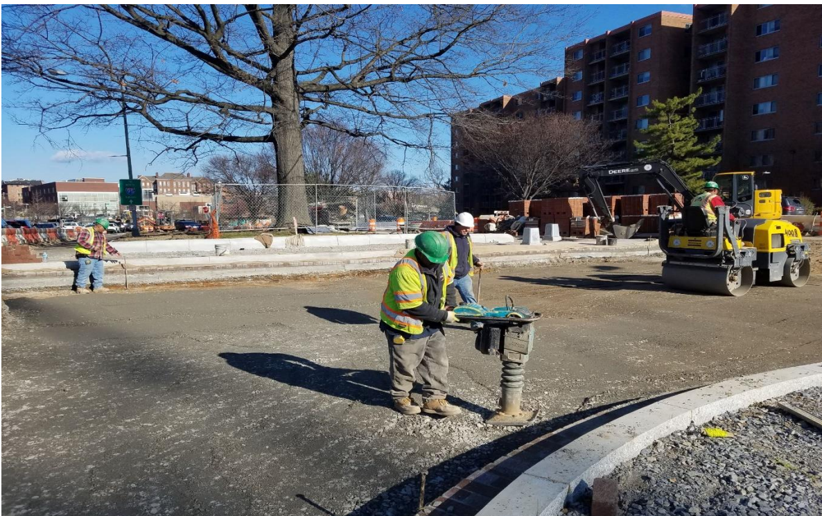
01/16/2020- Compaction to subgrade at intersection of I St. & 2 nd St. & NJ Ave. NW. (NE View)
