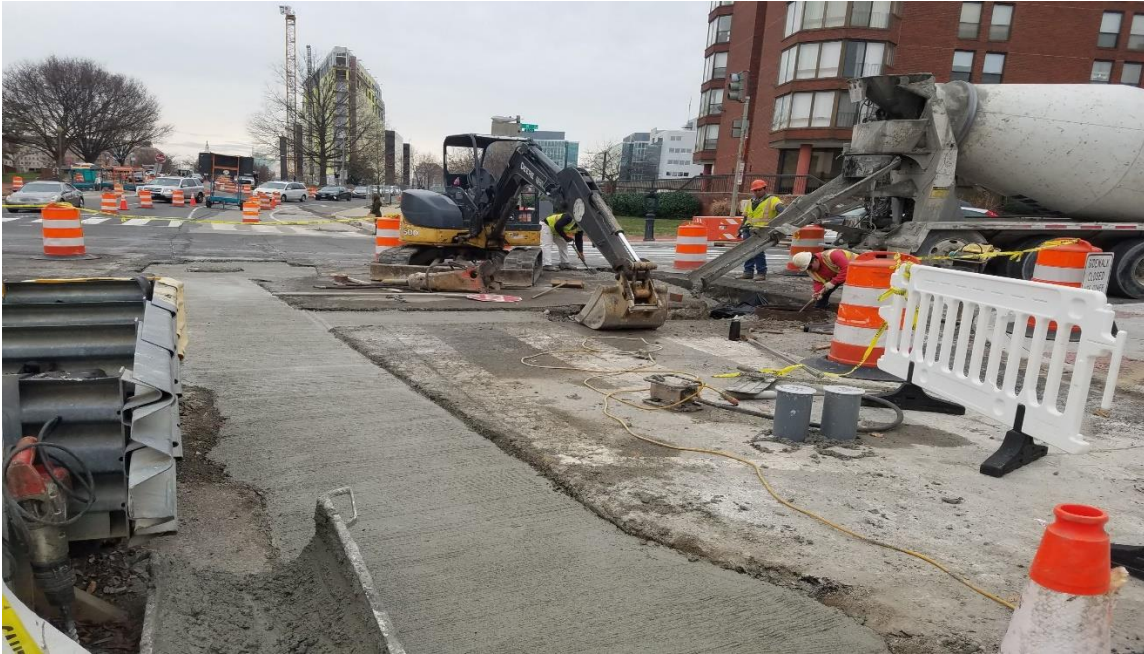
01/13/2020- Repair/replace PCC base over utility cuts at NJ Ave. & K St. NW (South View)
