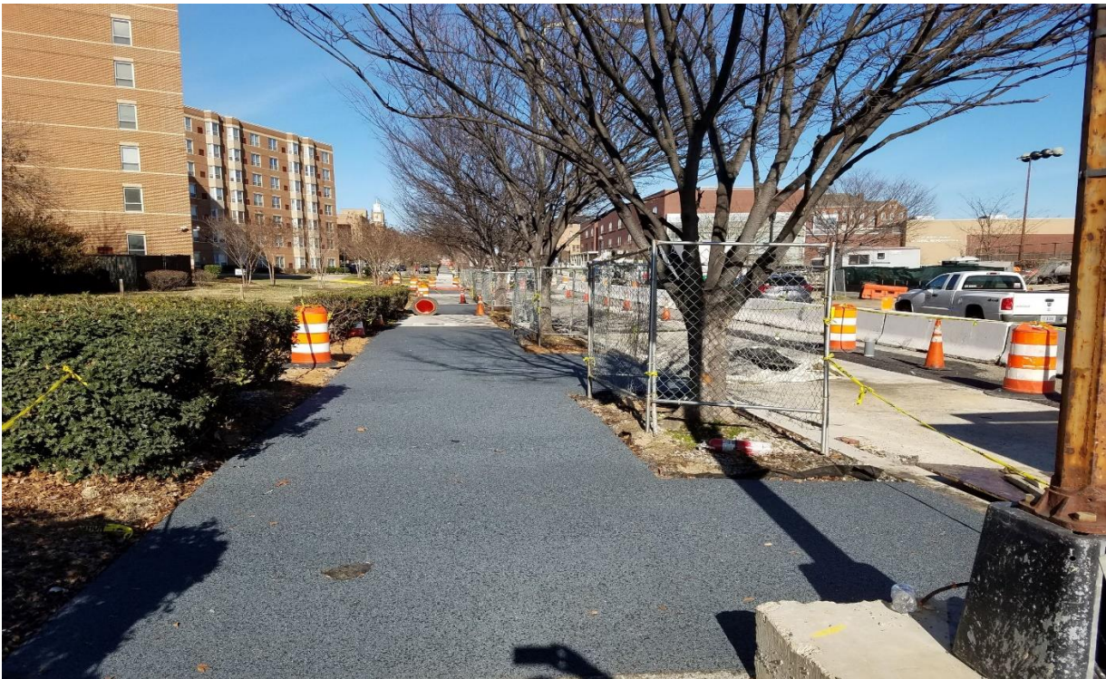
01/17/2020- Flexi pave sidewalk area replaced at West side of NJ Ave. between K & L St. NW.
