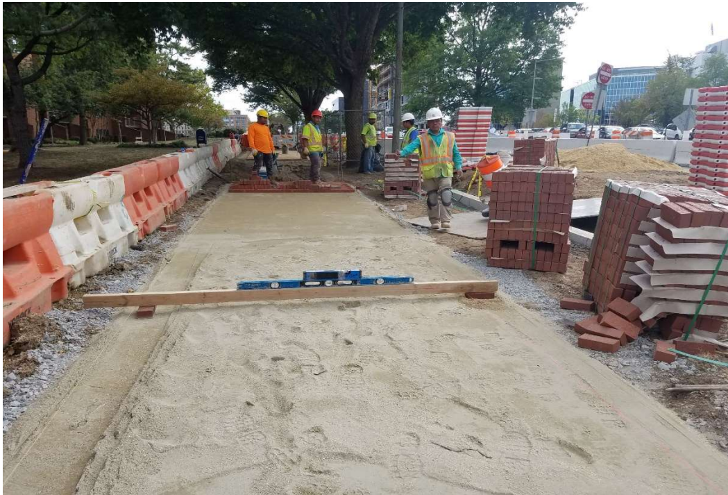
09/17/2019 – Grade checking for section of sidewalk needs flexi pave at NJ Ave. NW b/n K & I St. NW
