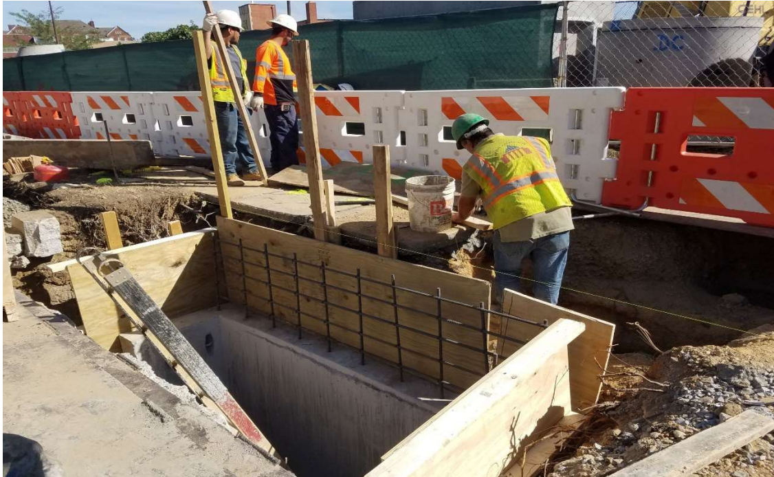
09/20/2019- CPDC modifying the catch basin Q3 at NE corner of NJ & K St. NW. (East view)
