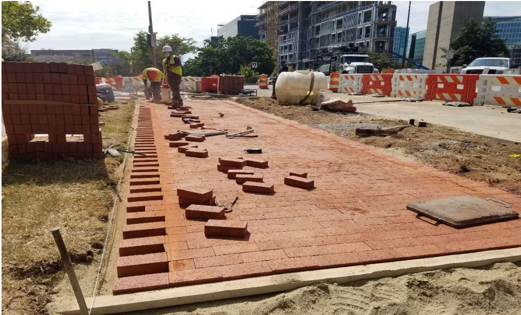
09/16/2019- Brick Sidewalk Construction at East side of NJ Ave. NW b/n K & I St. NW (South View) Picture No. 2
