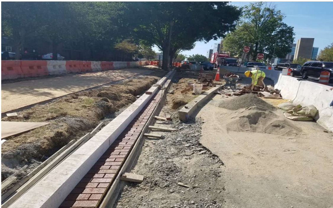
09/20/2019- Granite Straight curb and brick gutter installed at East side of NJ between K & I St. NW.
