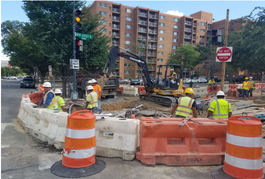
09/18/2019 – Excavation to install Wheelchair/Bicycle Ramp at SE corner of NJ & K St. NW (East View)
