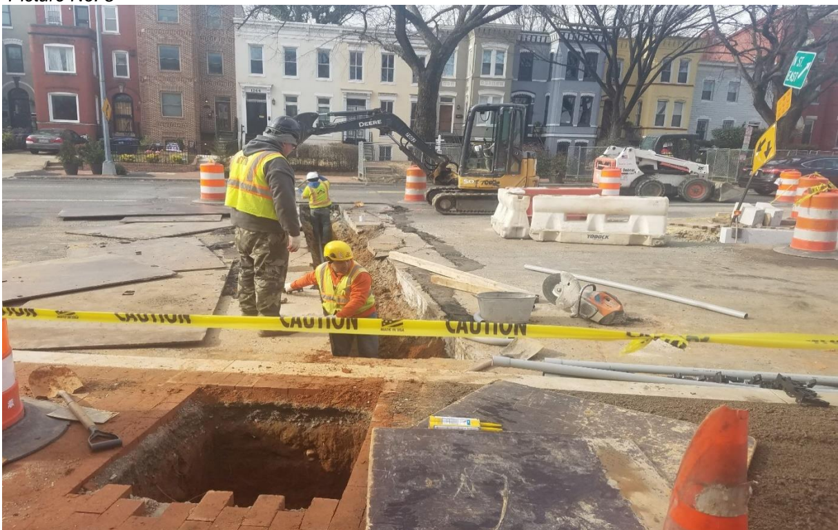
01/30/2020- Conduit installation for streetlight laterals at NJ Ave. NW b/n Morgan & N St. (West view)
