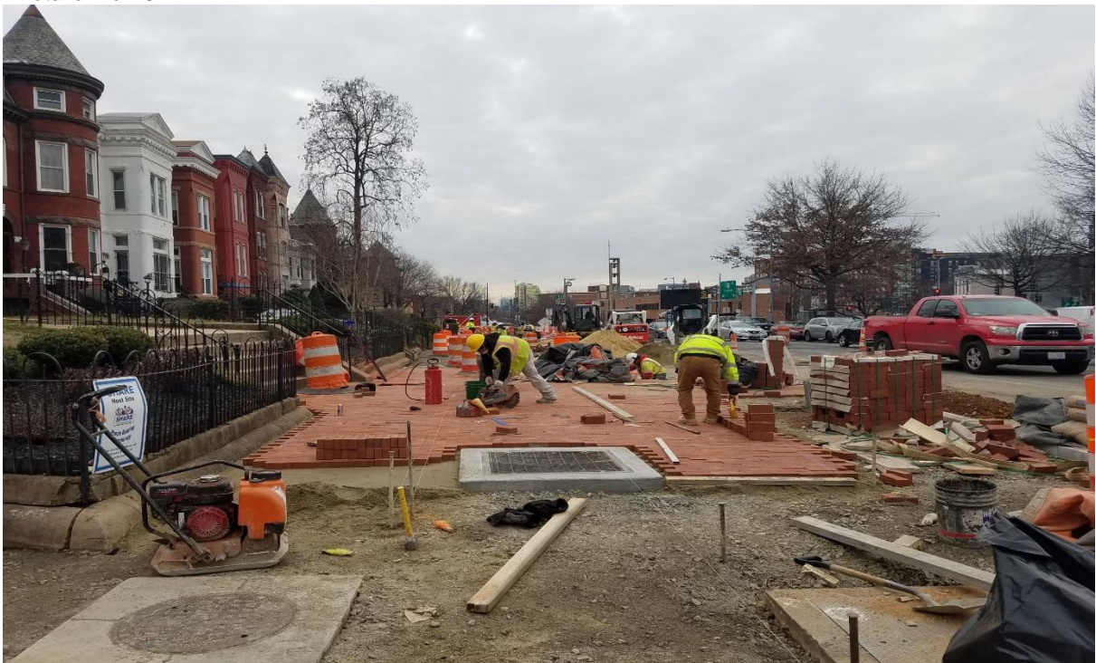
01/31/2020- Brick sidewalk construction at East side of NJ Ave. b/n Morgan & M St. NW. (South View)
