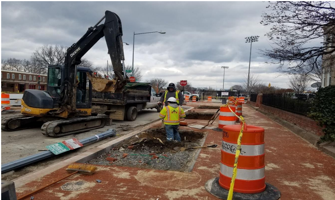
01/27/2020- Preparation of planting/tree boxes at East side of 3 rd St. b/n Morgan & N St. NW. (N. view)
