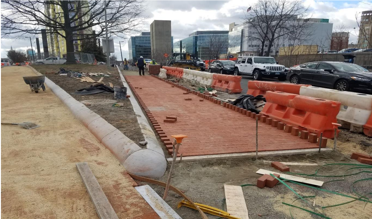
01/28/2020 – Brick sidewalk construction at East side of 2 nd St. b/n NJ Ave & I St. NW (South View) Picture No. 4
