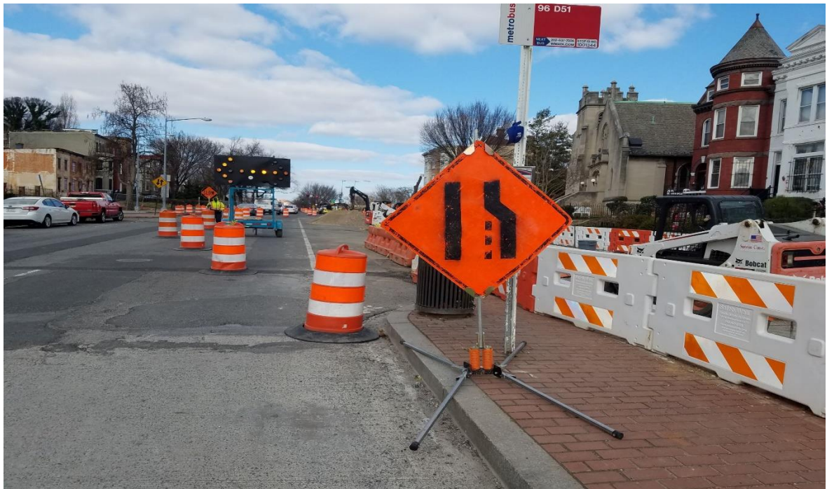
01/29/2020- MOT set up at New Jersey Ave. NW north of New York Ave. (North View)
