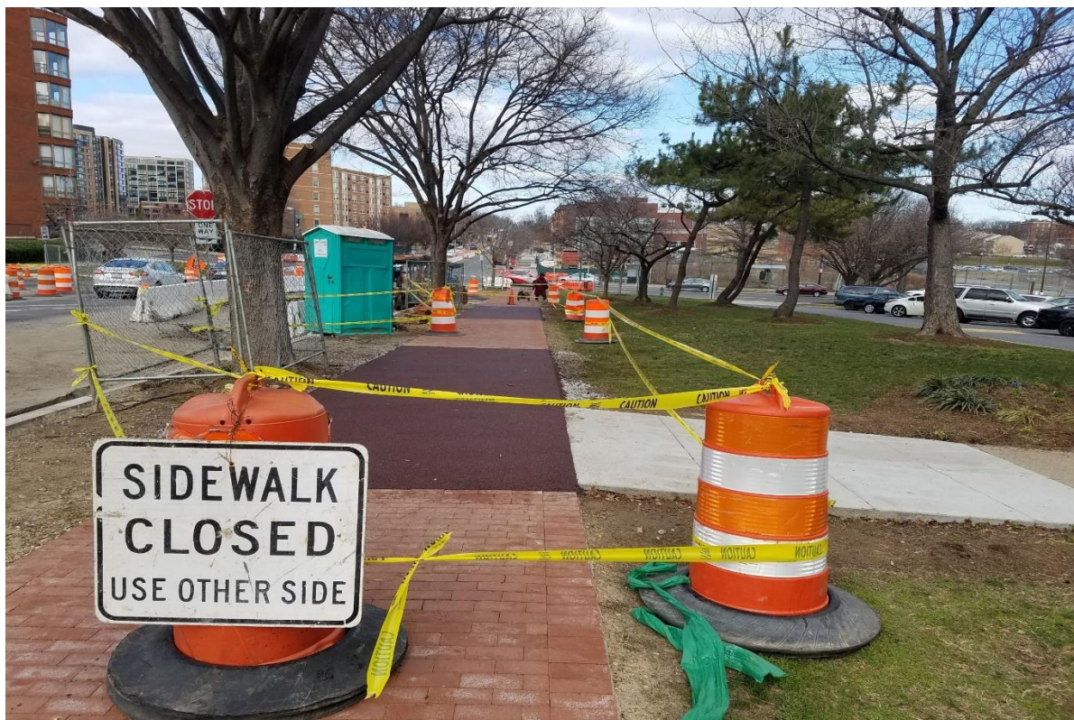
01/29/2020 - Flex pave sidewalk repaired at East side of NJ Ave. b/n K & I St. NW. (North view)
