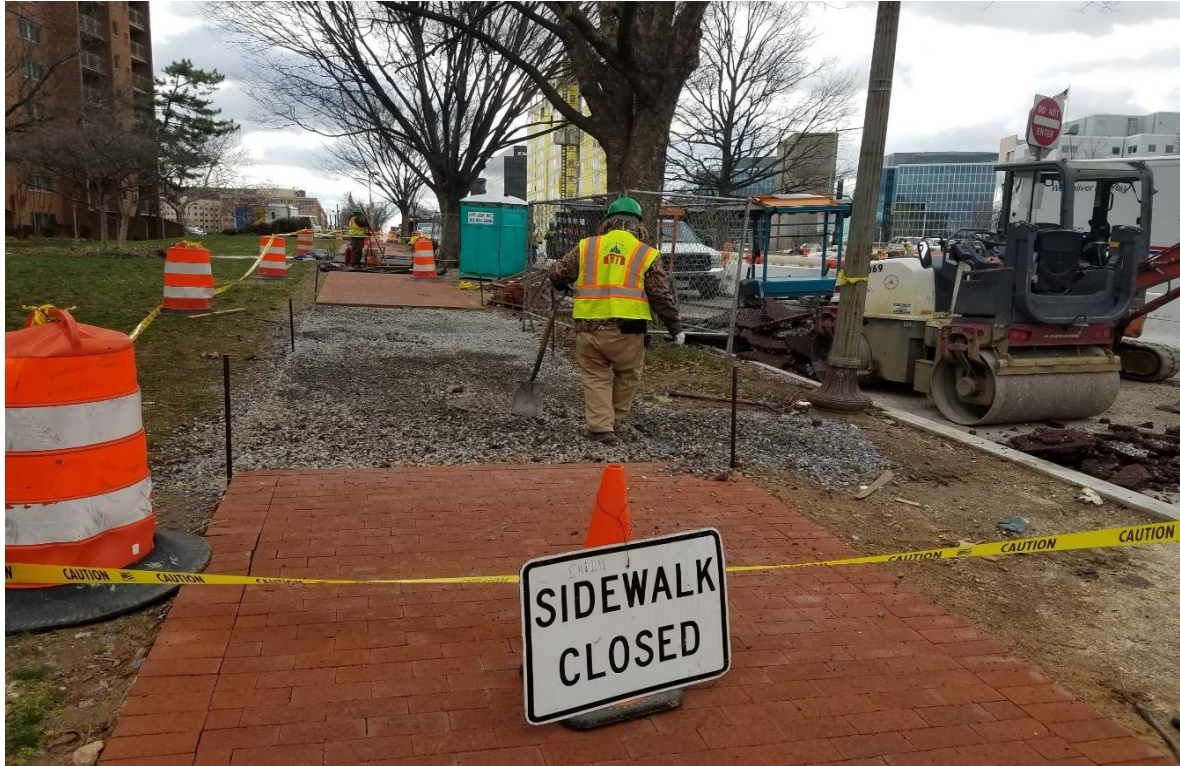
01/28/2019- Removal of deficient flex pave at East side of NJ Ave. b/n K & I St. NW. (South view) Picture No. 6
