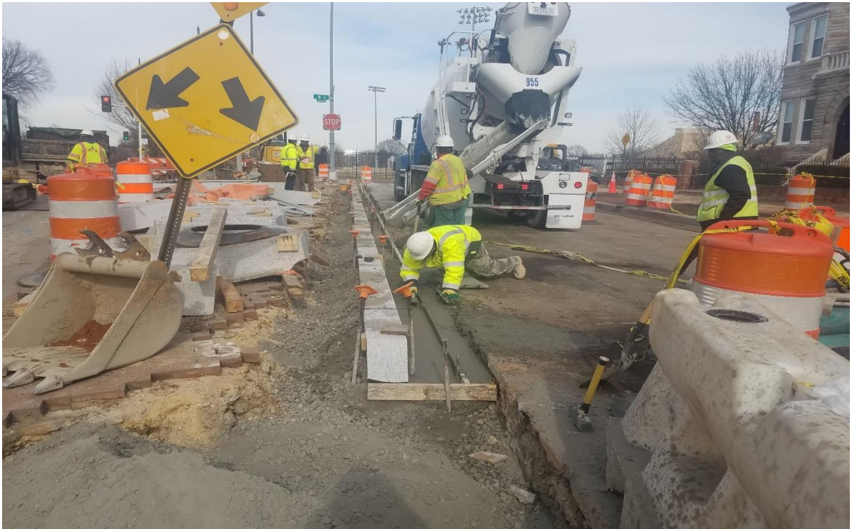
01/30/2020- PCC base construction along gutter line at NJ Ave. NJ b/n Morgan & N St. (North view)
