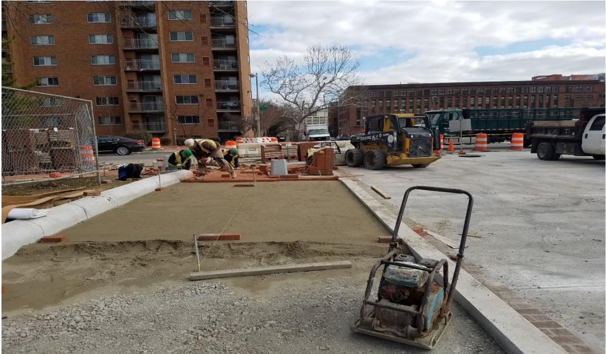
01/29/2020- Brick sidewalk Construction at North side I St. b/n 2 nd & NJ Ave. NW. (East View)
