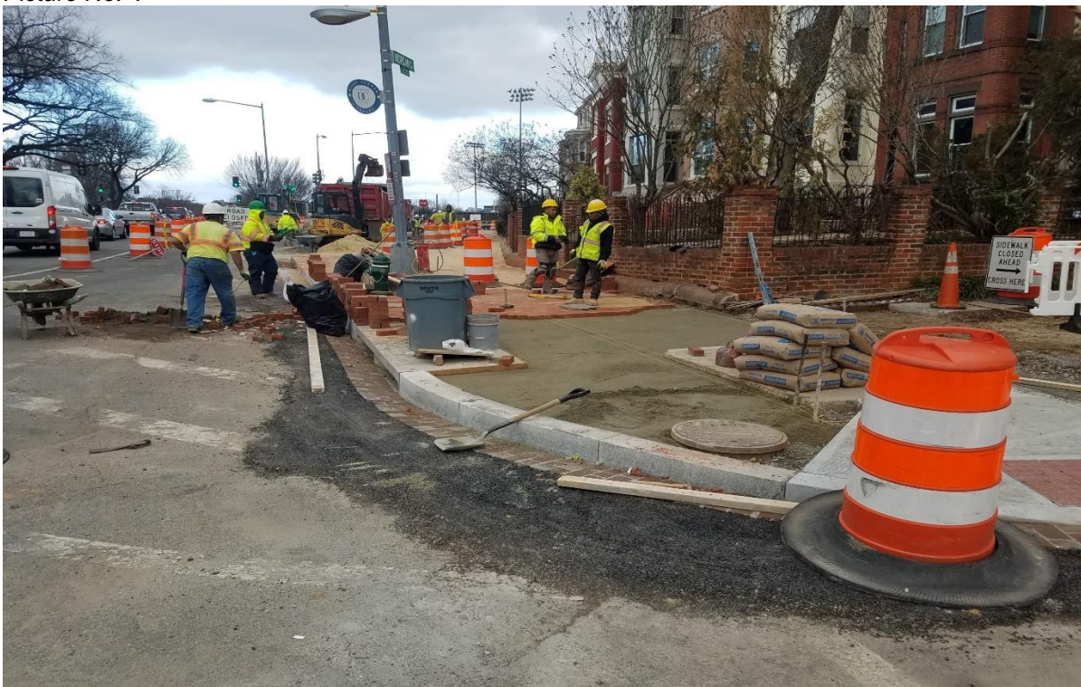
01/28/2020- Brick sidewalk construction at East side of 3 rd St. b/n Morgan & N St. NW. (North view)
